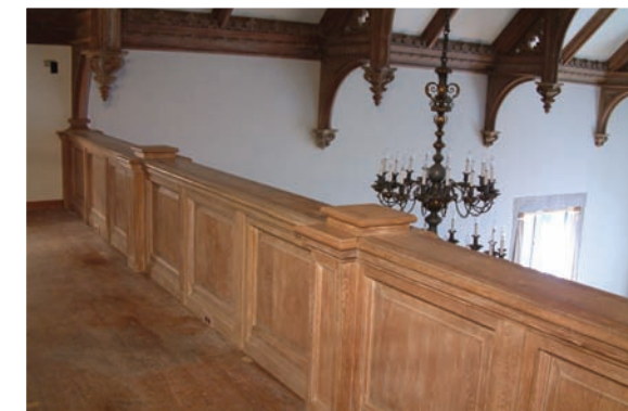
2009 and 2010 the first two phases of a three phase project were completed to restore the Minstrel Gallery overlooking the Living Room.
